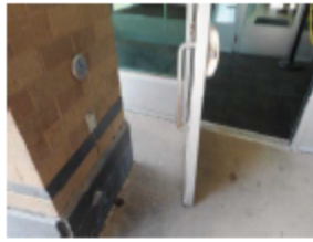
Photo 1: The east entry to the courts building currently provides a power operated door opener. The clear floor space for the button is currently within the arc of the door swing.
