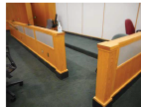
Photo 5: There are 2 courtrooms with jury seating. An accessible route is provided to both levels of the jury seating; the main level is deep enough to allow for a wheelchair space. This is a good example of accessibility.
